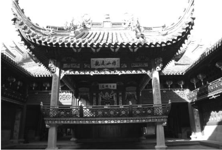
Figure 10. Theater Stage Roof after Remedy
