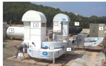
Figure 6. Photograph of the liquid desiccant system: 1 – absorber/dehumidifier; 2 – desorber/regenerator; 3 – air ducts; 4 – fan; 5 – rotary air/air heat exchanger; 6 – control cabinet; 7 – solar collector field; 8 – hot water storage tank. (Gommed and Grossman, 2007)
