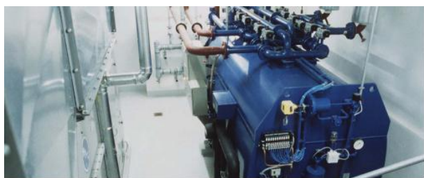
Figure 11. 70 kW adsorption-chillers in a hospital, in Freiburg, Germany (Henning, 2007)
